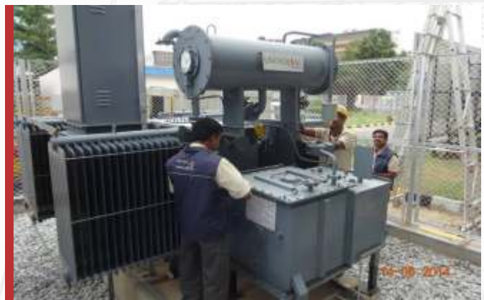
Oil filtration and BDV test
